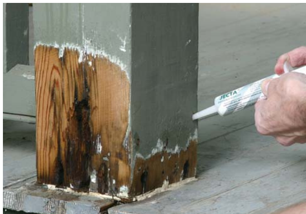
Figure 1. A painter's 5-in-1 is the perfect tool to carve into rot-damaged wood and excavate the black, punky detritus (top). After the worst of the damage has been removed, a solution of powdered borate and water is sprayed on the affected surfaces to kill the rot organism (center). To quickly attack deeply buried rot, a borate gel is injected into a few small holes that have been drilled into the center of the wood (above).
