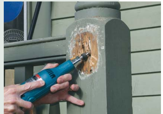
An alternative to fortifying rot-softened wood fibers with an epoxy consolidant is to remove all of the suspect material with a power tool — such as the die grinder shown here, which is equipped with a 1/2-inch-diameter core box bit.
