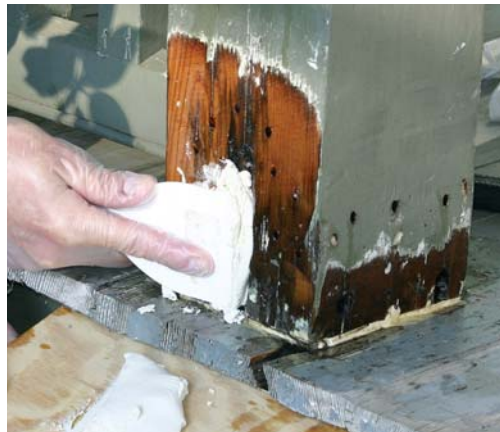
Figure 4. Using a plastic putty knife, the author presses the epoxy paste firmly into the crevice, then wipes the surface smooth (left). After the epoxy has fully cured, he begins the tooling process by shaving down the rough spots with a Surform plane (below).
