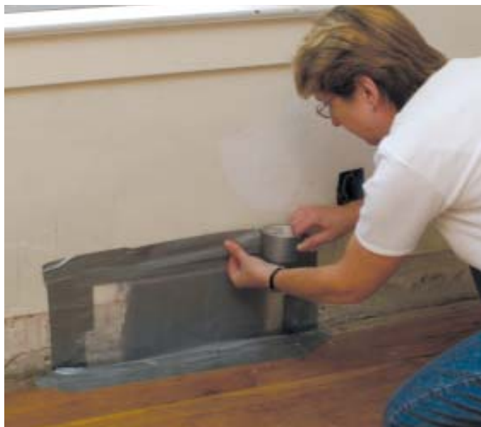
Figure 1. Sealing off this cold-air return duct ensures that job-site dust does not get blown throughout the house.
