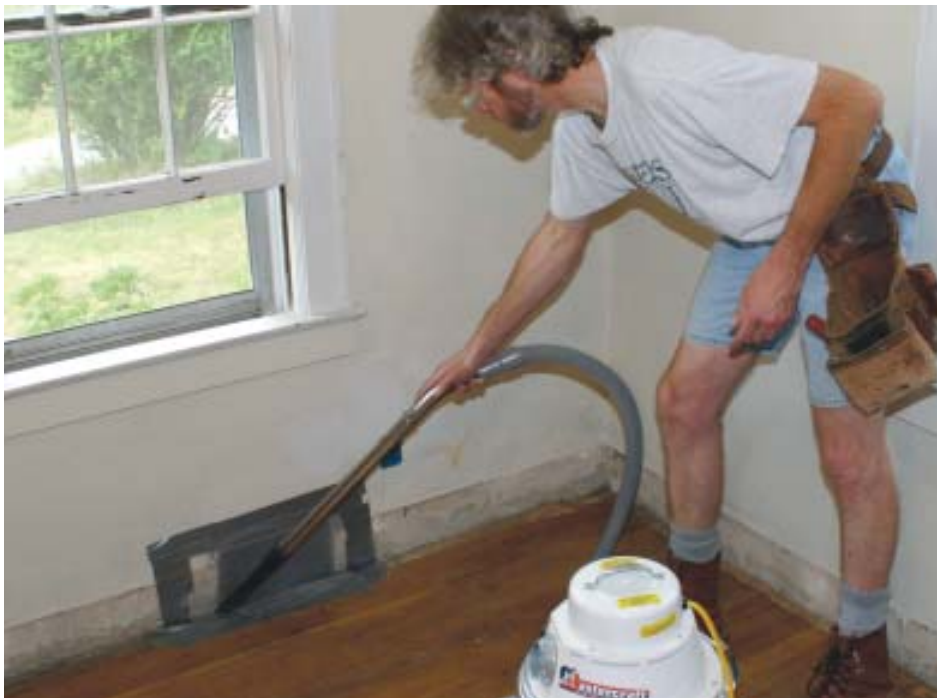
Figure 4. After the dirty work is done, all surfaces and crevices should be slowly and thoroughly vacuumed with a HEPA vac.
