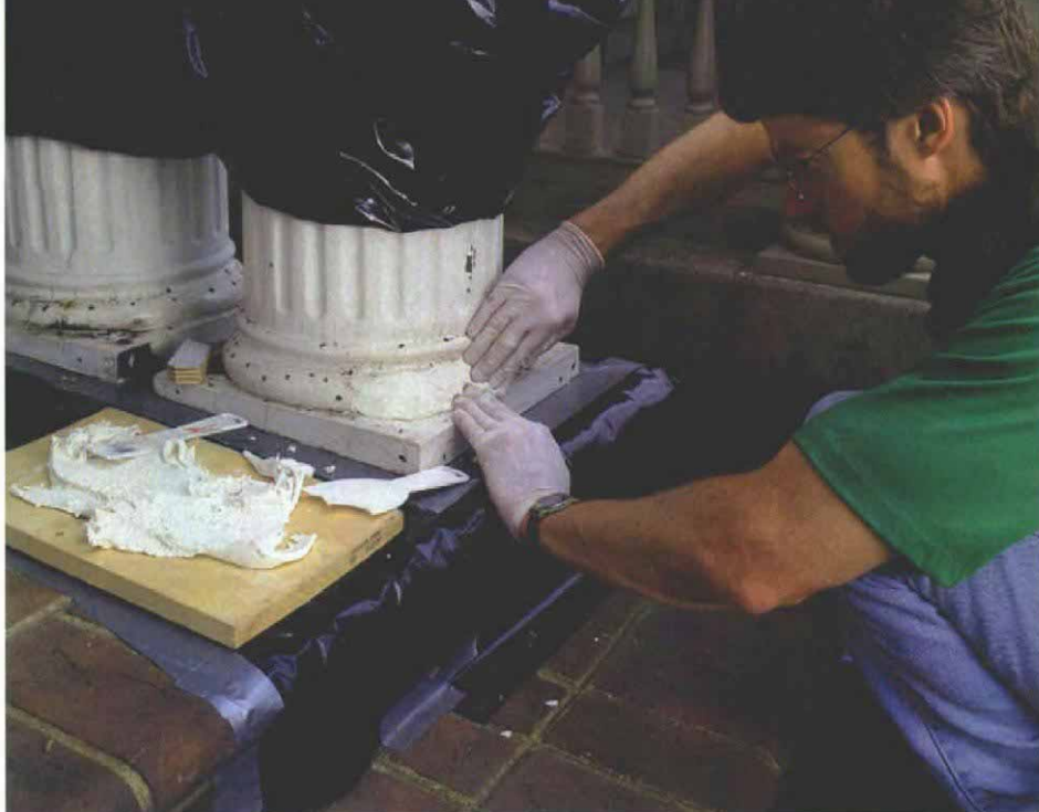
The rest of the hole is filled by hand. Epoxy paste is packed into the repair by hand until the entire gap is filled.
