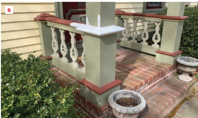
With two coats of paint and an annual inspection, this repair should last indefinitely (9).
